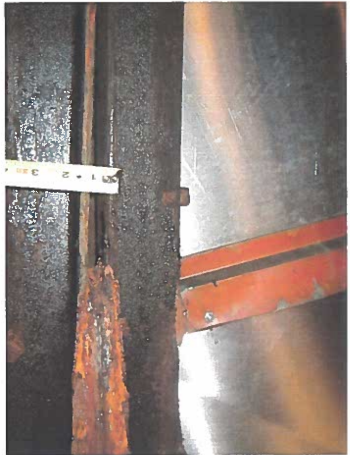
Figure 8 Close-up of rust jacking.
