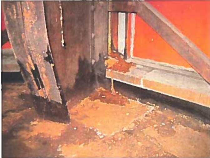
Figure 11 Rust piling up behind bottom of truss.
