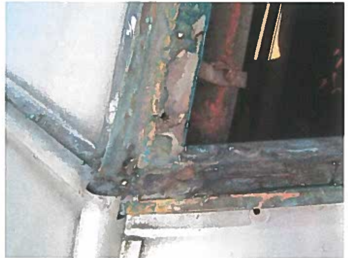
Figure 9 Note brittle sealant around framed opening.
