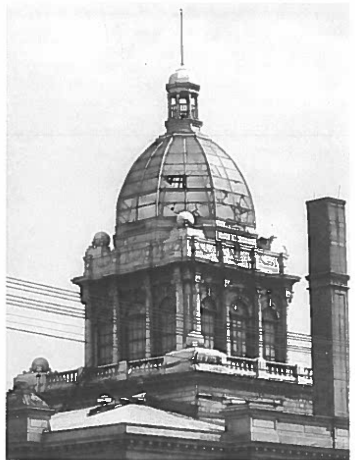
Figure 2 The 1950 storm damage.
