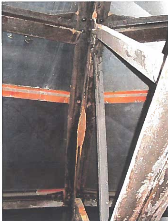
Figure 7 Rust jacking at upper truss.
