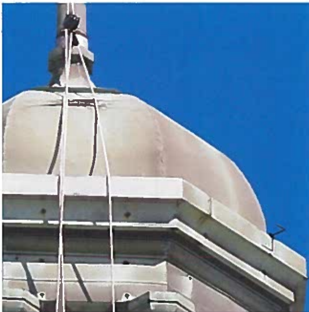
Halyards rubbing on dome and pulled taught to edge of cornice.
