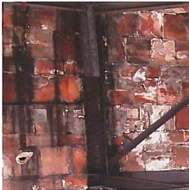
Extensive water staining and efflorescence of structural clay tile. Note heavy corrosion of steel column supporting dome truss
