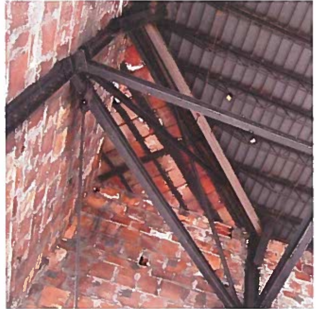
Water staining and efflorescence on structural clay tile walls and corner ceiling.
