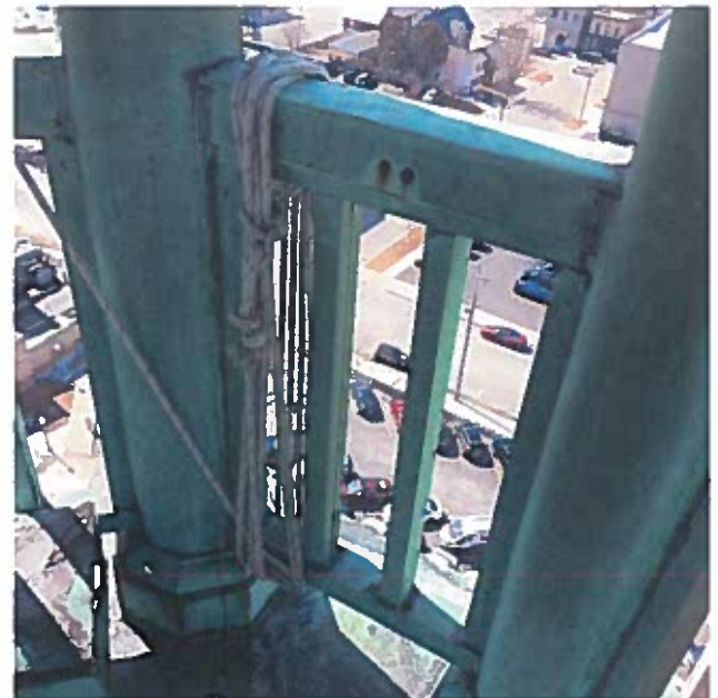
Halyards tied around guardrail. Note rusted anchors for missing cleat on rail.
