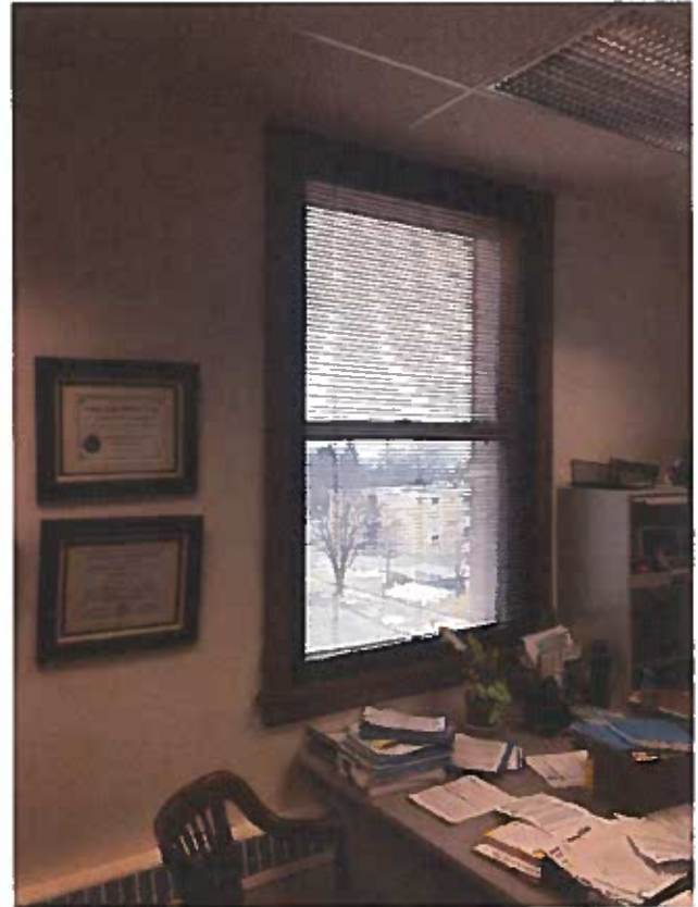
Typical window at interior. Note how dropped ceiling cuts off top of window. The spandrel panel is above the ceiling line.
