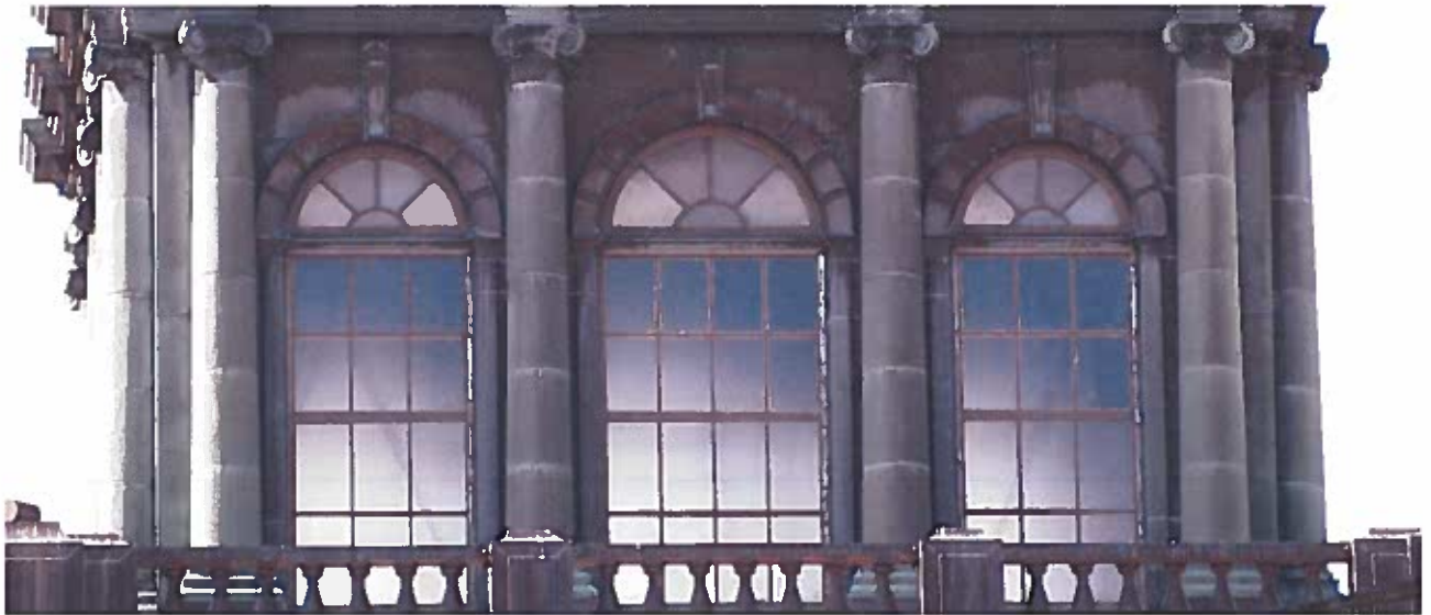
The clerestory windows; the half round sunburst windows are original with original glass.
