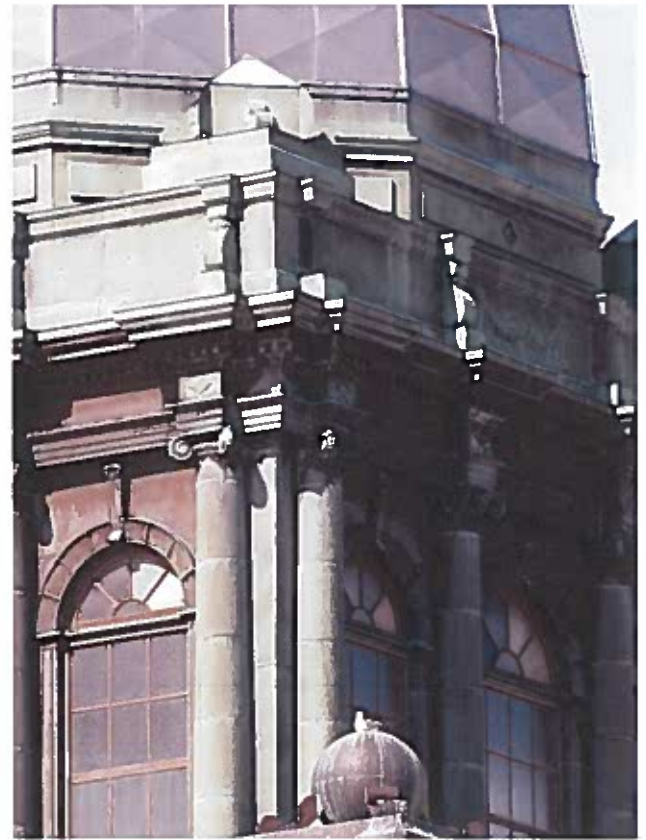
May, 2022: Extensive missing ornament and the simplified window frames of the 1950s repairs.
