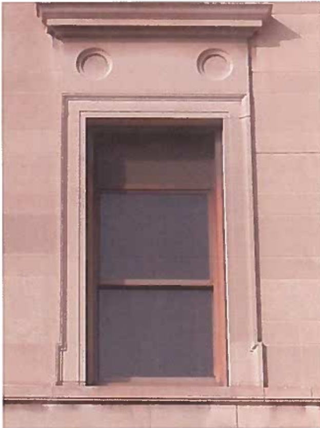
Typical aluminum exterior window, note fading of dark bronze anodizing. Reduced sash size allows for the insertion of an opaque spandrel panel.
