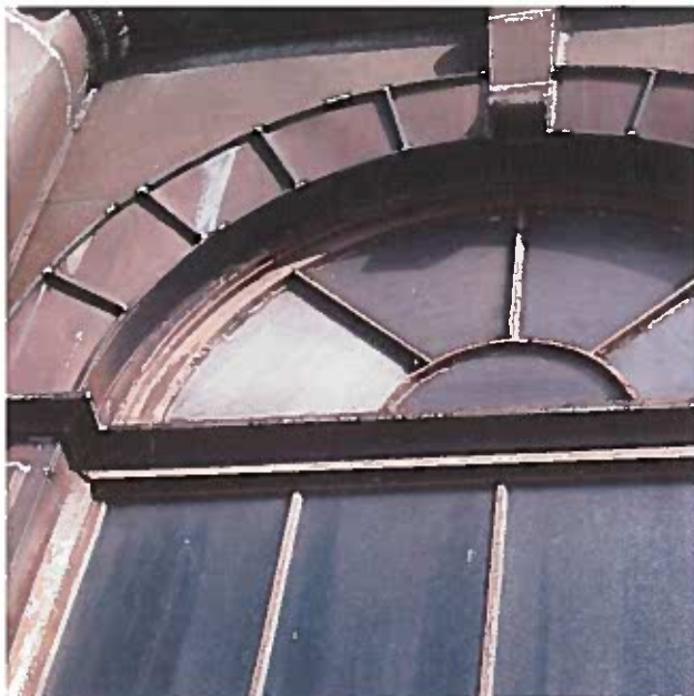
The frame and muntins of the original sunburst windows are thicker than the replacement sash below.
