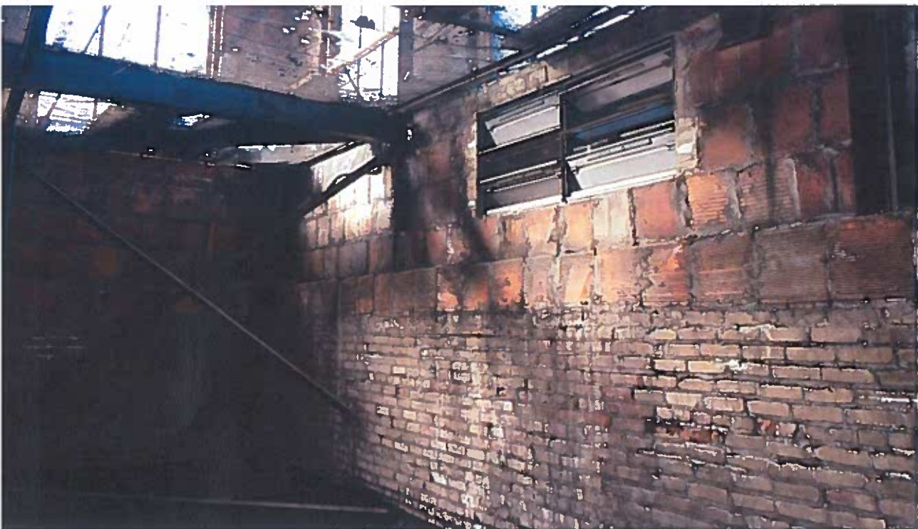
View of the clerestory just below the debris screen. Limited efflorescence and spalling brick indicate a minimum amount of water infiltration of the past 100 years. Note barometric pressure louver below center window.
