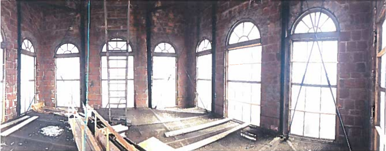
Interior of clerestory. Note structural clay tile, steel columns, wood bracing of windows, wood catwalk, and debris screen over lower cross bracing. The ship ladder in the center leads to the dome.
