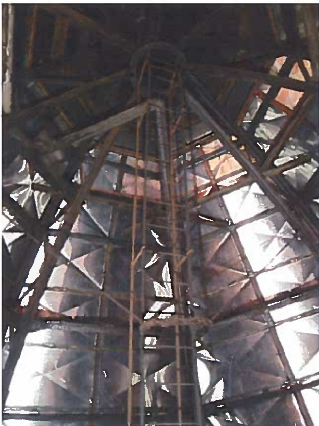
Dome structural trusses connect to a compression ring at top of dome. Note ladder to lantern through ring.
