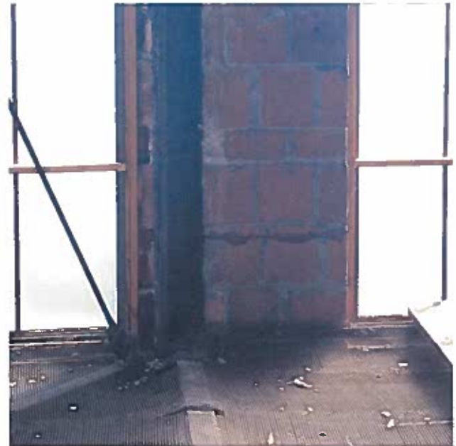
Broken infill tile between window and steel column.
